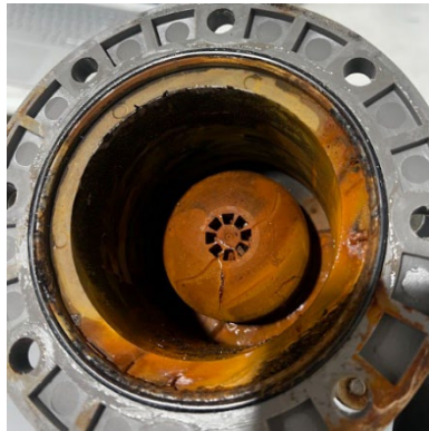
Wet end water intrusion
