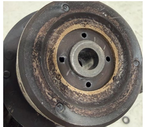
Inspect the impeller assembly for melted plastic, worn bushings, impeller damage, etc.
