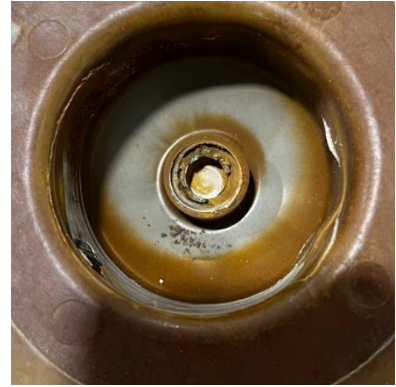
Barrier damaged and melting
