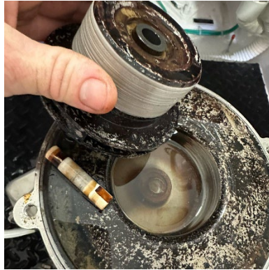
Impeller magnet damage due to bushing failure
